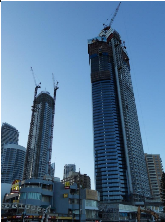
55 + storey apartments, Surfers Paradise, Gold Coast, Australia (Smallwood, 2011)
