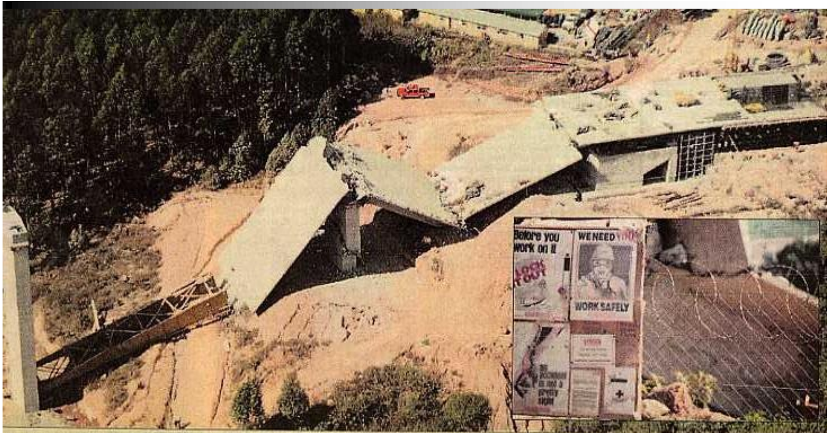
Disaster area: The construction of a road bridge near Injaka Dam turned into disaster when it collapsed, instantly killing 12 people and injuring 15. Two of the injured died later. Insert - A reminder to workers of the dangers of working on a construction site. Full update on page 2. Photographs by Raymond Travers.
