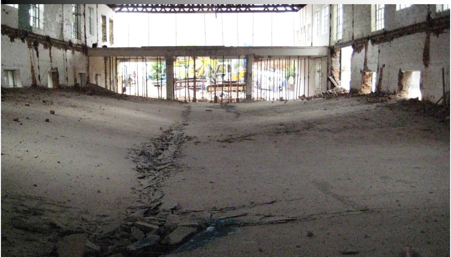
Stellenbosch Collapse (Anonymous, June 2008)
