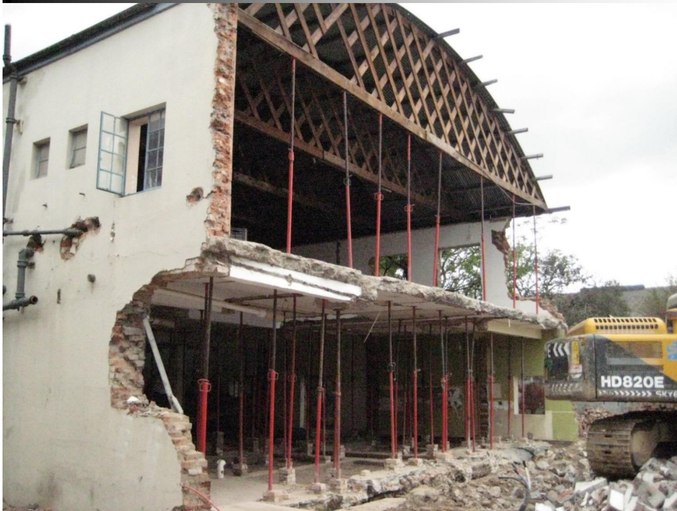
Stellenbosch Collapse (Anonymous, June 2008)
