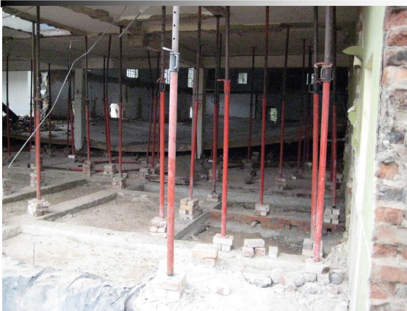
Stellenbosch Collapse (Anonymous, June 2008)
